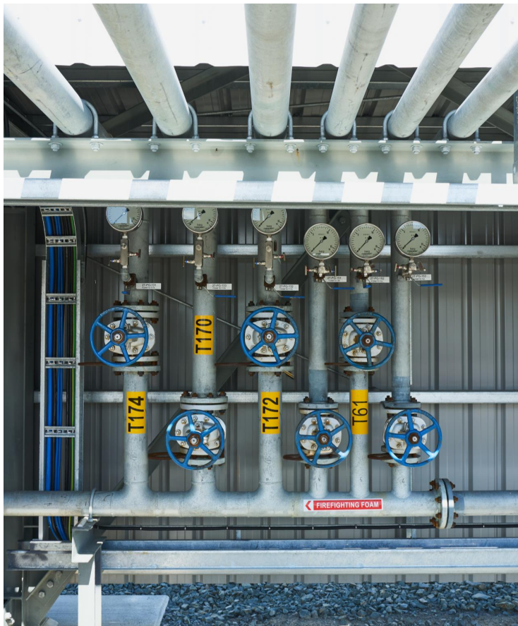
Petrol tank farm firefighting manifold
