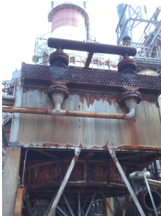
Figure 5: An Example of a Fanfan Cooler in A-Block showing the Tube Plugs removed and significant corrosion to the fan cowling and header box.
