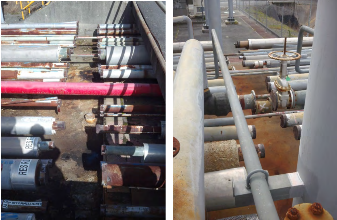
Figure 6: Example of Air-Gapped Piping. Left: A-Block and Off-plots, Right: D-Block and Off plots - 20/08/24
