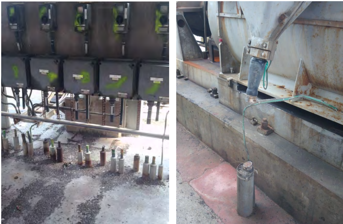
Figure 7: Typical Example of Cable 'Air-Gapping', Left: Power/Instrument Cables to Hazardous Area Junction Boxes, right: Power Supply to Electric Motor – 20/08/24.
