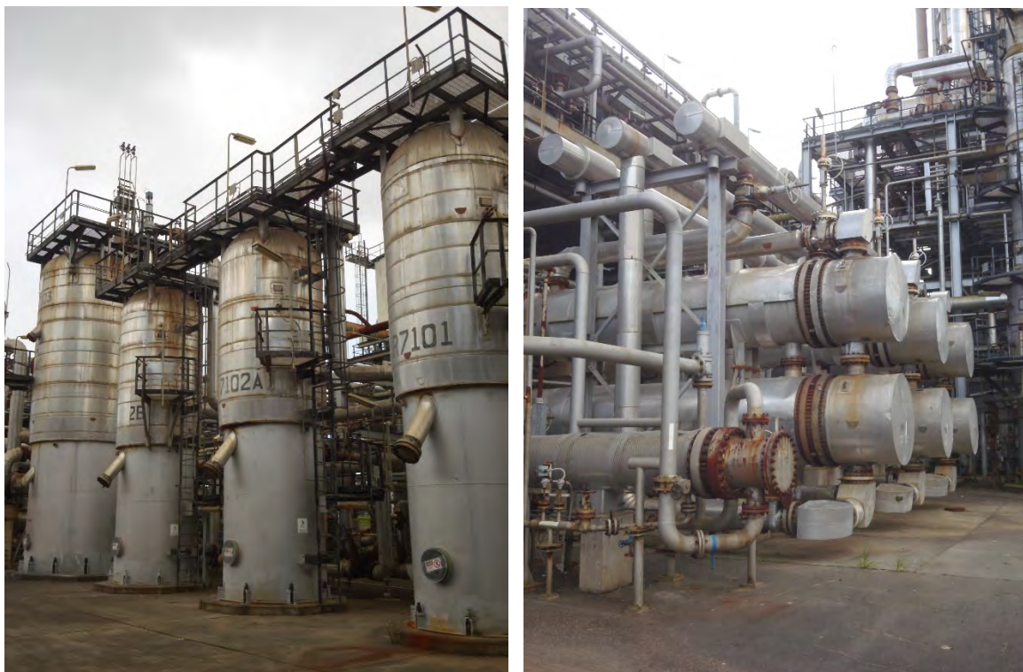
Figure 10: Equipment under Preservation in C-Block. Left: HMU Reactors. Right: ADIP-X Shell & Tube Exchangers remain assembled.
