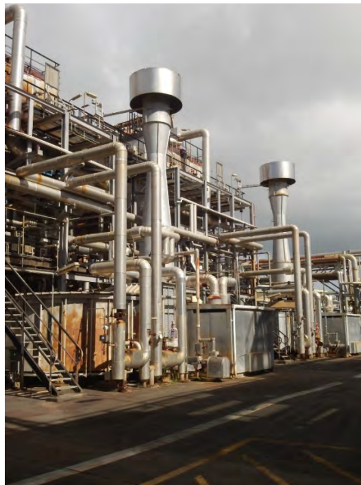
Figure 17: Two of the Three Steam Boilers in B-Block
