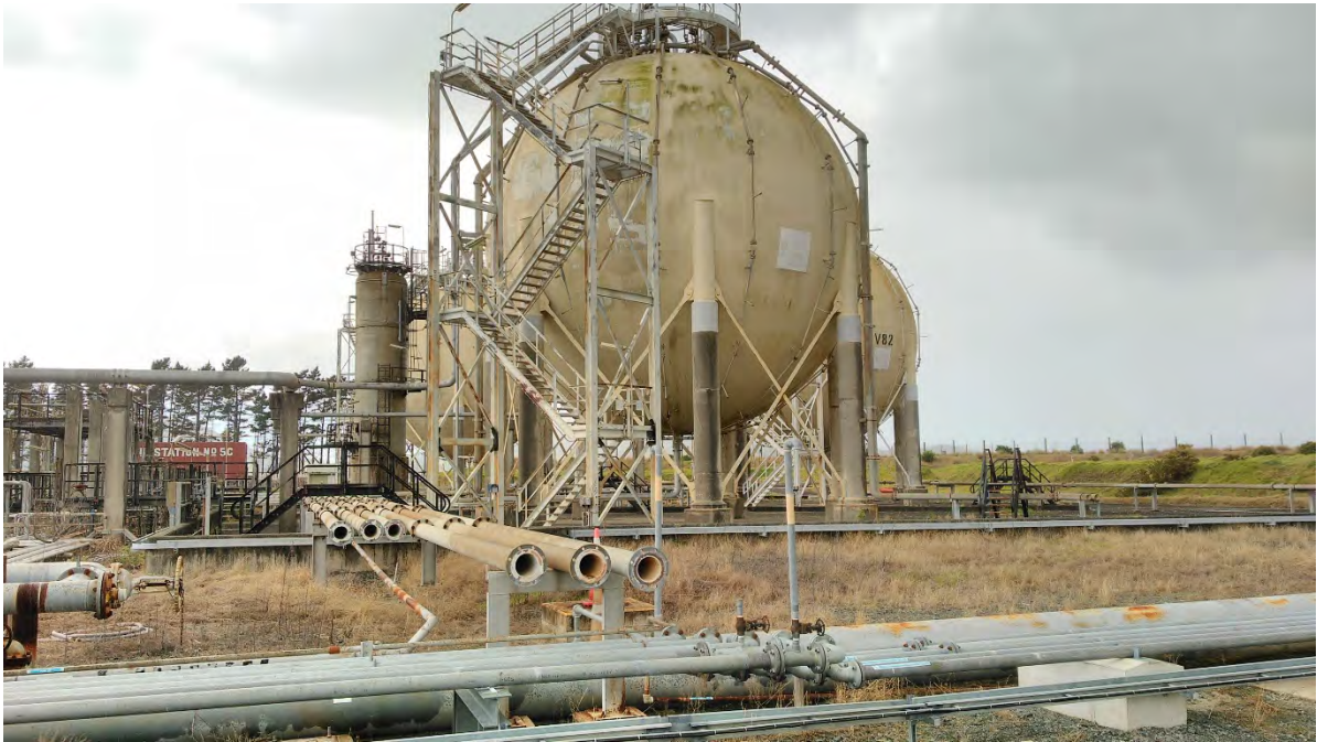
Figure 14: The piping to and from the Butane Sphere's located in the offplot areas has been demolished as part of the conversion to a terminal.
