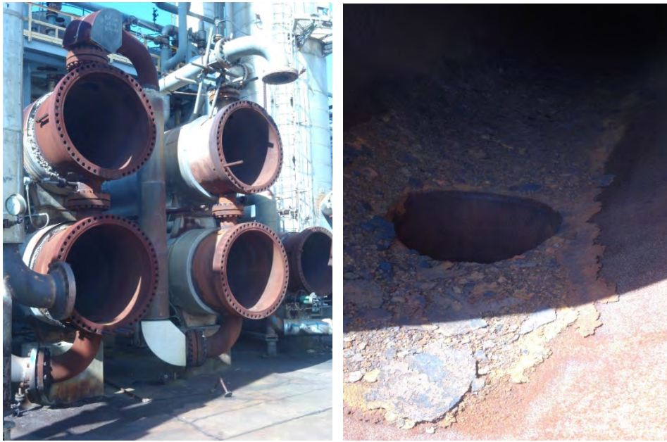
Figure 4: Example of Rust Scale build-up within Exchanger Shells in the 250-unit. – 20/08/24.
