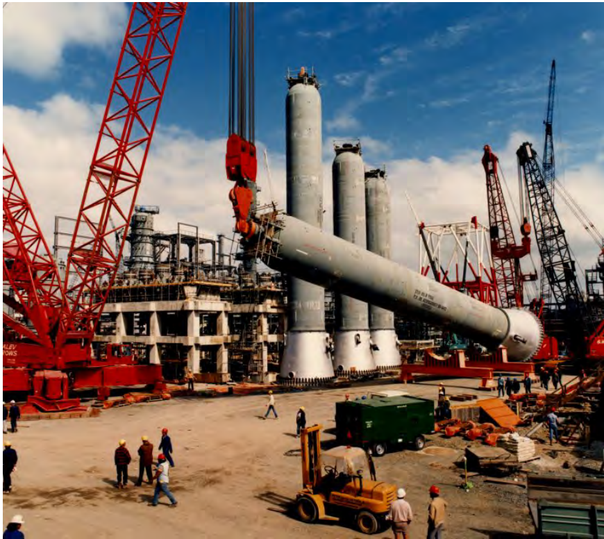
Figure 2: Hydrocracker R-7502 being lifted into place during the 1980's Refinery Expansion. Photo courtesy of: https://channelnz.com/who-we-are/our-history/
