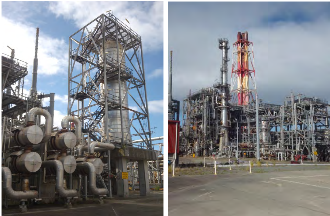
Figure 9: Typical Example of the Equipment in D-Block. Left: Shell & Tube Exchangers & equipment remains Boxed up. Right: General Photo of D-Block.
