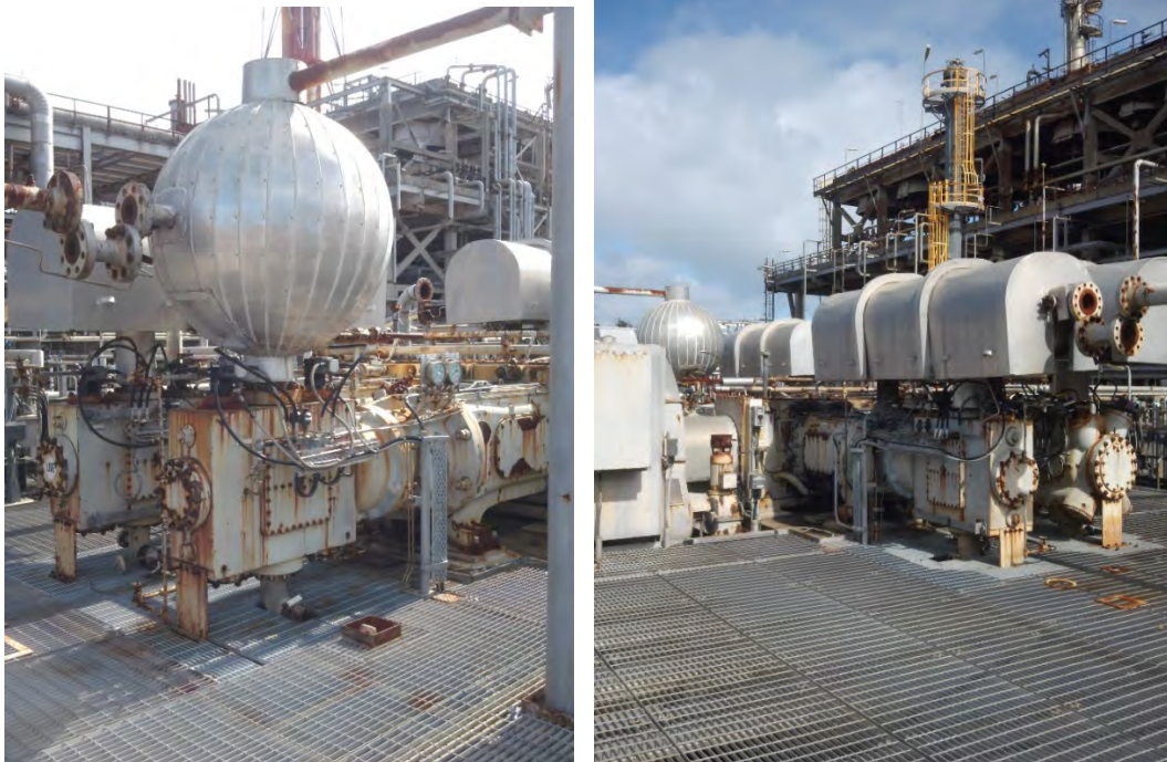
Figure 18: Four Stage Reciprocating Hydrogen Compressors
