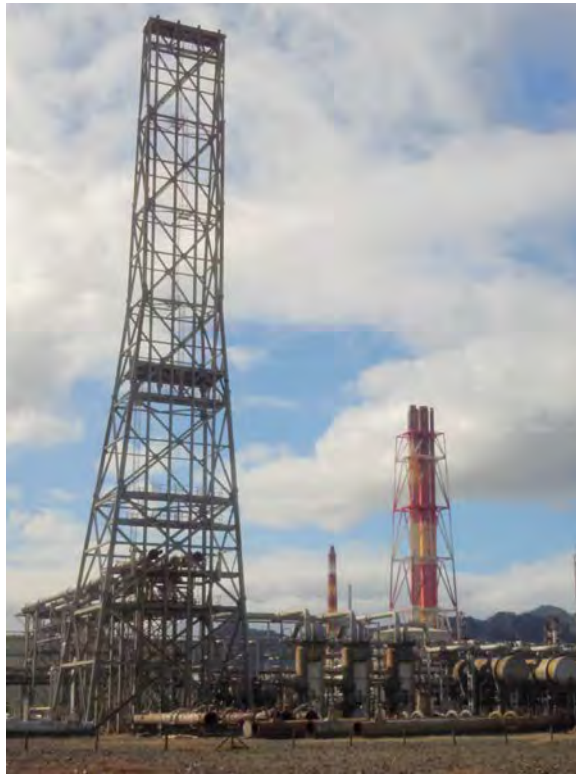
Figure 8: Flare System showing the Elevated Flare sections removed and Disassembled at Grade - 20/08/24.
