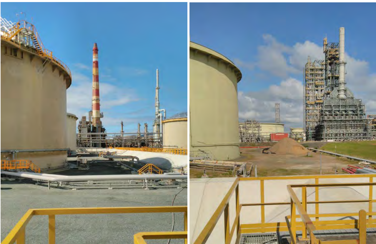
Figure 13: An Example of an Upgraded Bund relative to an Existing. Left: Existing Crude T04 Converted to Jet A1 located in the newly upgraded C3 Compound. Right: Crude Tank T05 currently decommissioned, piping can be seen to be removed, secondary containment is no longer compliant.
